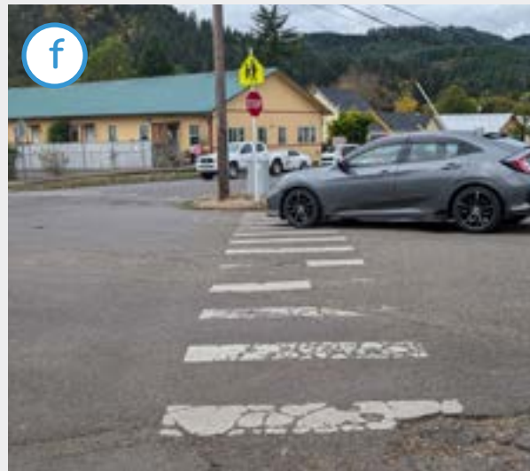
Cars come to a rolling stop or inch out onto the diagonal crosswalk on the west leg of the intersection of Moreland Avenue and Main Street. Additionally, the crosswalks are faded, and there are missing curb ramps at this intersection.
