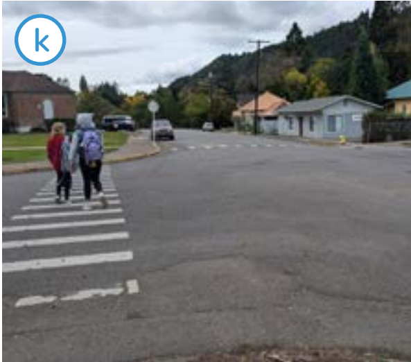
Many crosswalk markings near both the elementary and high school are very narrow.
