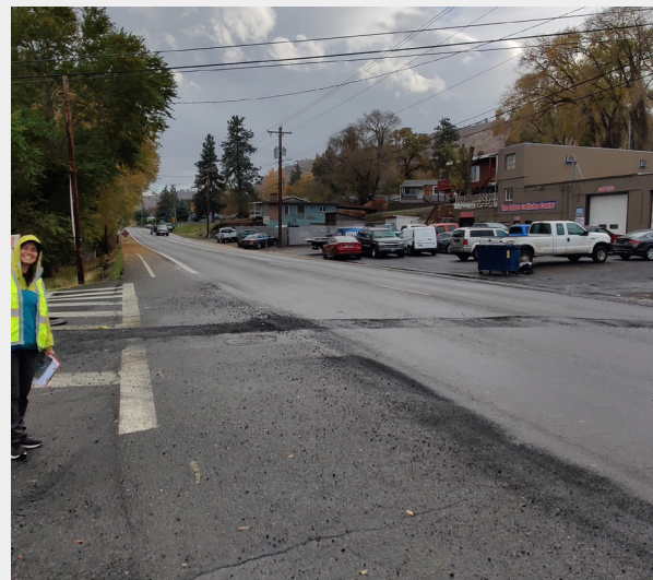
No curb ramps exist on either side of the crosswalk at Hostetler St and 10th St.
