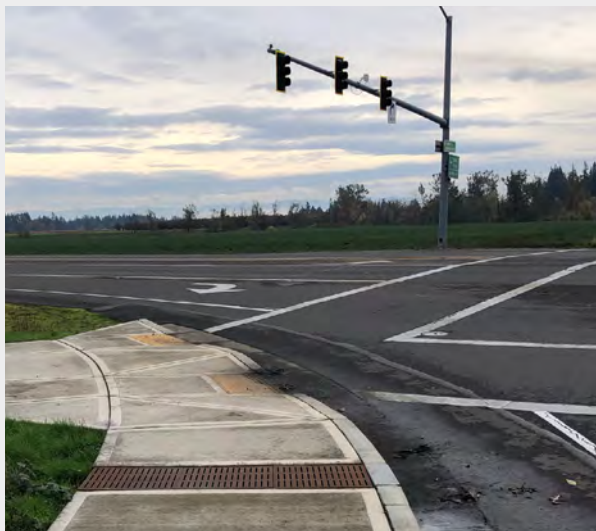
The curb radius on the northwest corner of Douglas Ave and Hwy 99E is wide. A narrower curb radius would encourage vehicles to slow down as they make the turn onto Douglas Ave and into Gervais.
