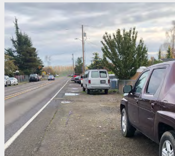
Sidewalk gaps along the south side of Douglas Ave create areas where students are walking through gravel parking areas with no curbs to separate them from the street.
