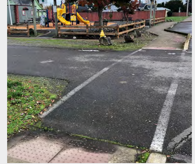
Sidewalks are in good condition and complete on the west side of 1st St between Ivy and Douglas. However, crosswalk markings along 1st St are not high-visibility and the paint is faded.
