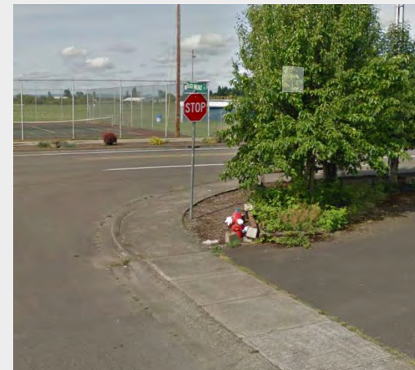
The NW corner of Douglas Ave at Black Walnut St does not include ADA-compliant curb ramps.
