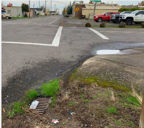
Existing crosswalk markings along Douglas Ave are not high-visibility, making them harder to see, especially during the winter or when it is dark. Curb ramps are also not ADA-compliant. For example, the above image shows the intersection of 3rd St and Douglas Ave.
